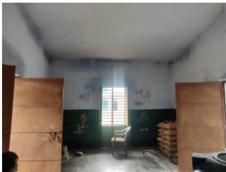
Inside ICDS Anganwadi Center Needing Repair
